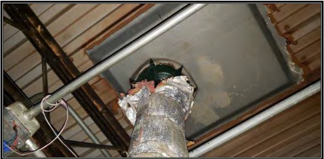
Photo 14: Non-ACM Fiberglass Drain Pipe Insulation
