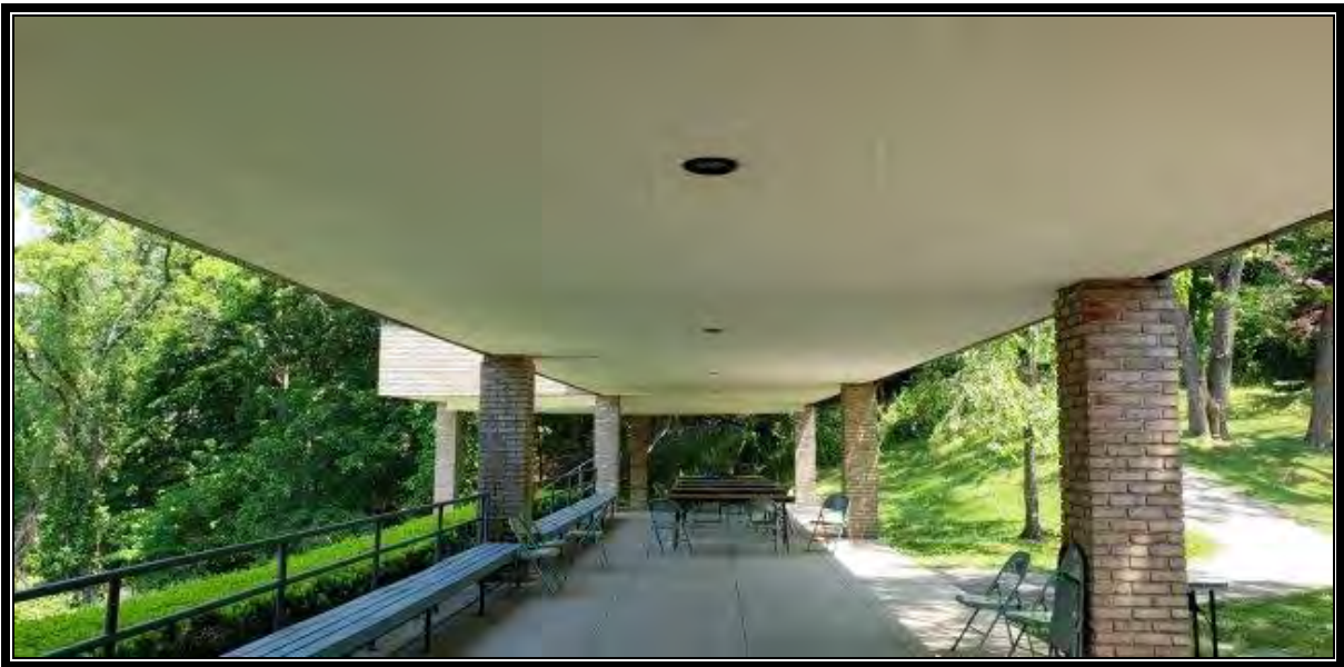
Photo 12: Non-ACM Scratch Coat on Exterior Soffit
