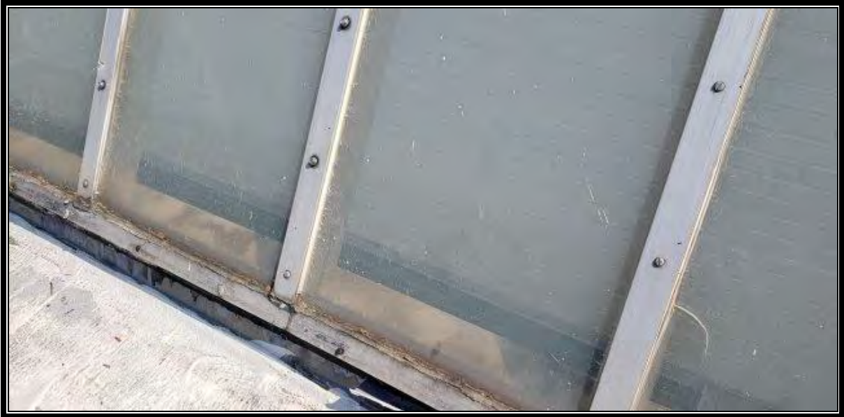
Photo 9: Non-ACM Skylight Panel Caulking, Beige and Skylight Old Caulking, White
