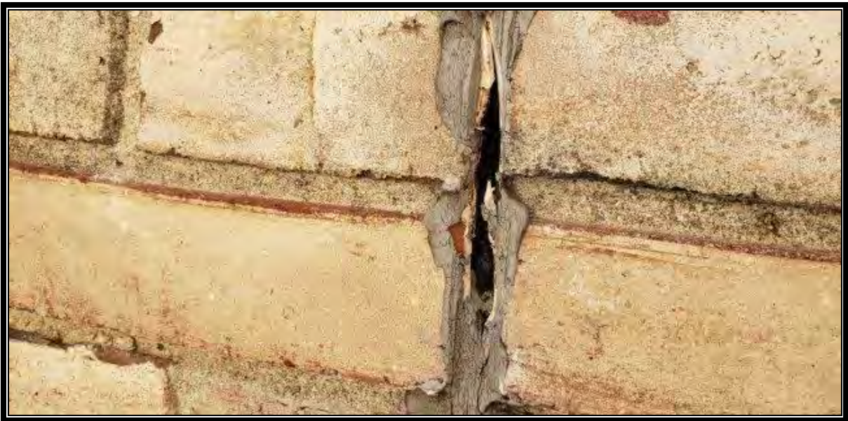
Photo 10: Non-ACM Wall Expansion Joint Tar, Black
