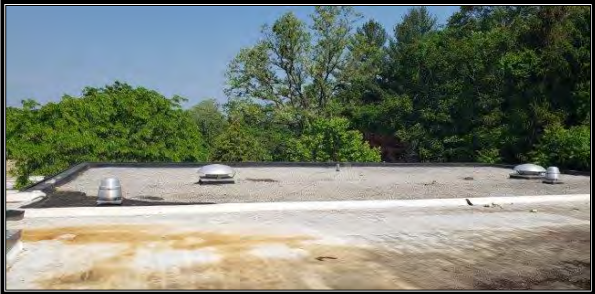
Photo 11: Non-ACM Tar on Roof Flashing, Black
