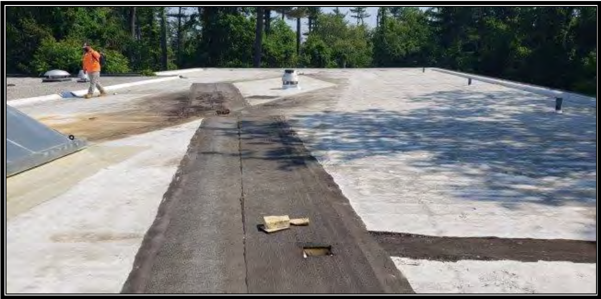
Photo 5: Non-ACM Roof Tar Patch
