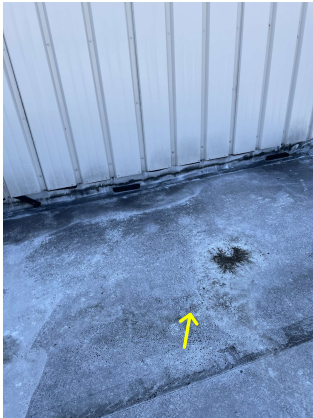
Top ply deterioration
