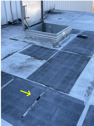
Dirt collection between pads
