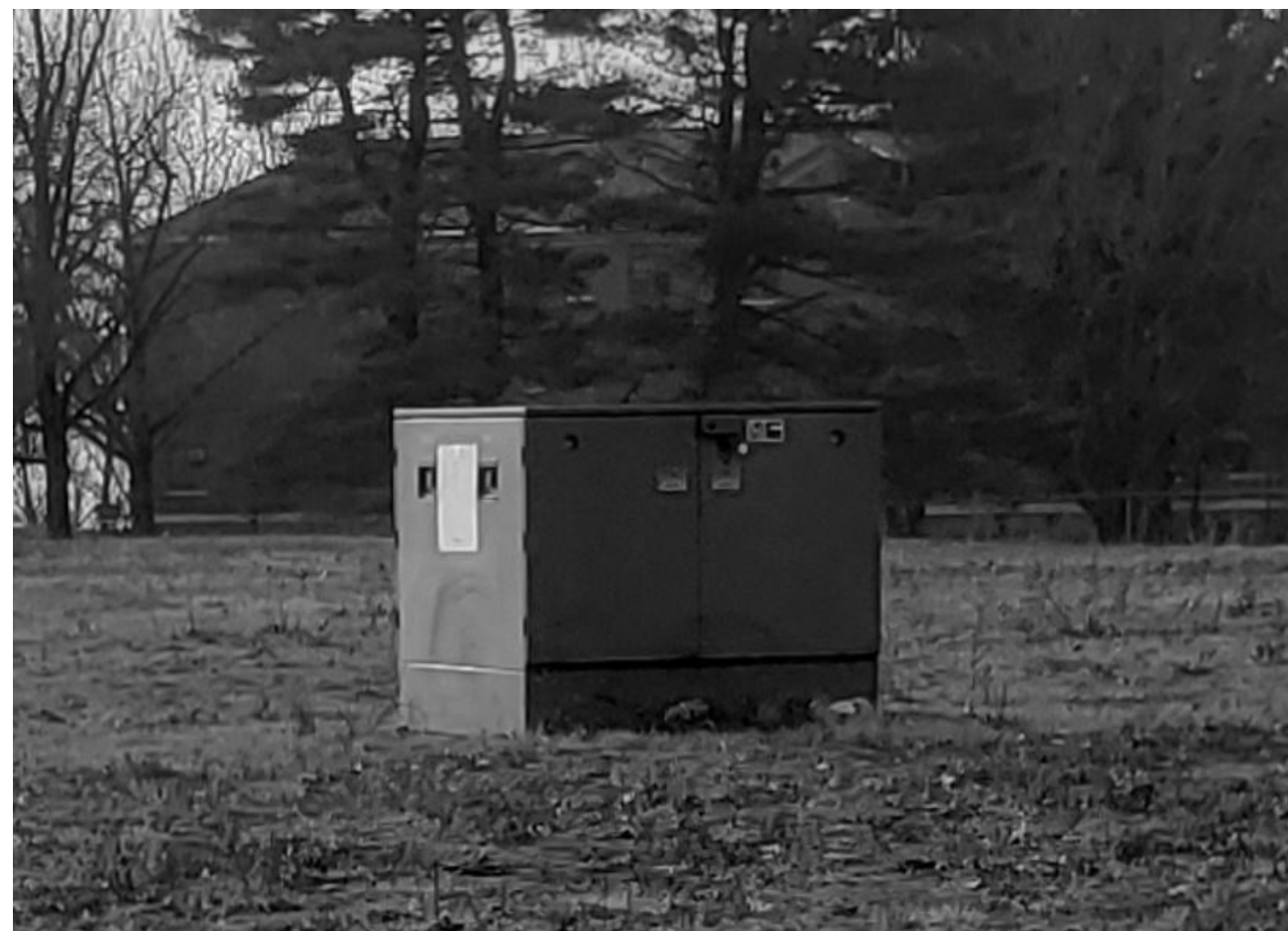
5 EXISTING SECTIONAL SWITCH, SS #12
