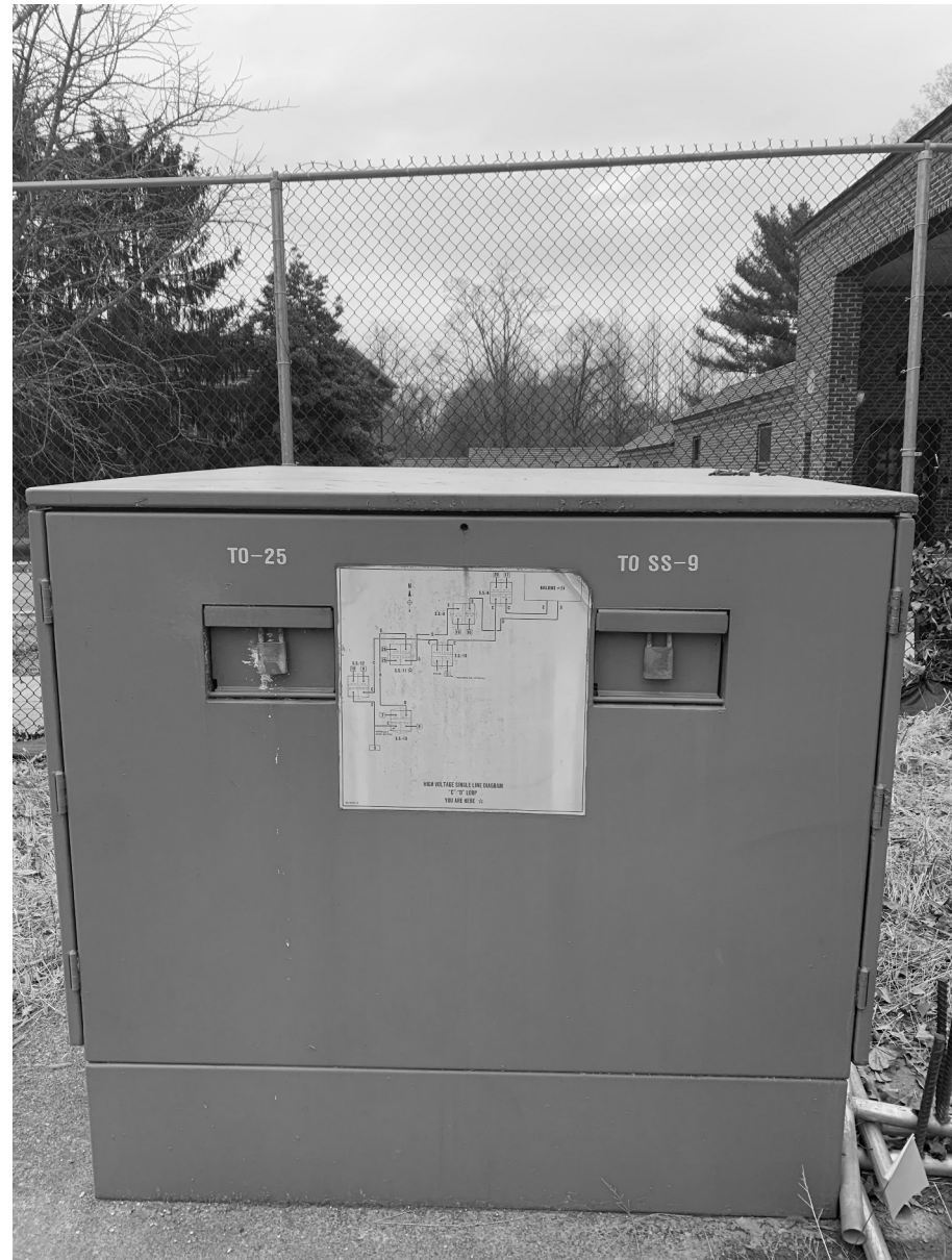
4 EXISTING SECTIONAL SWITCH, SS #11
