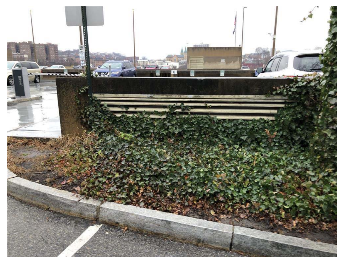
4 OVERGROWN VEGETATION INTO LOUVER D0.6 Not To Scale
