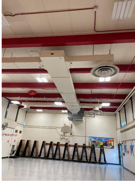
No Duct Insulation
