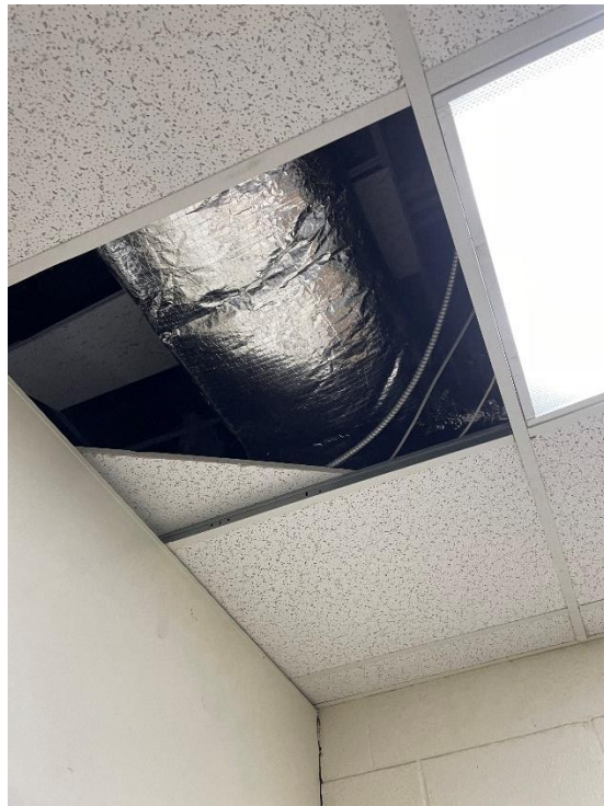
2x4 Fissured Ceiling Tile
