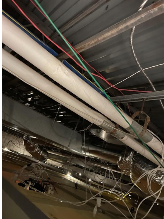
Fiberglass Pipe Wrap
