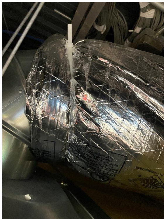
Flex Duct System
