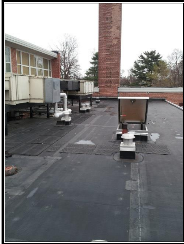
Photograph 5: Chimney Flashing Caulking & Pitch Pocket Tar.
