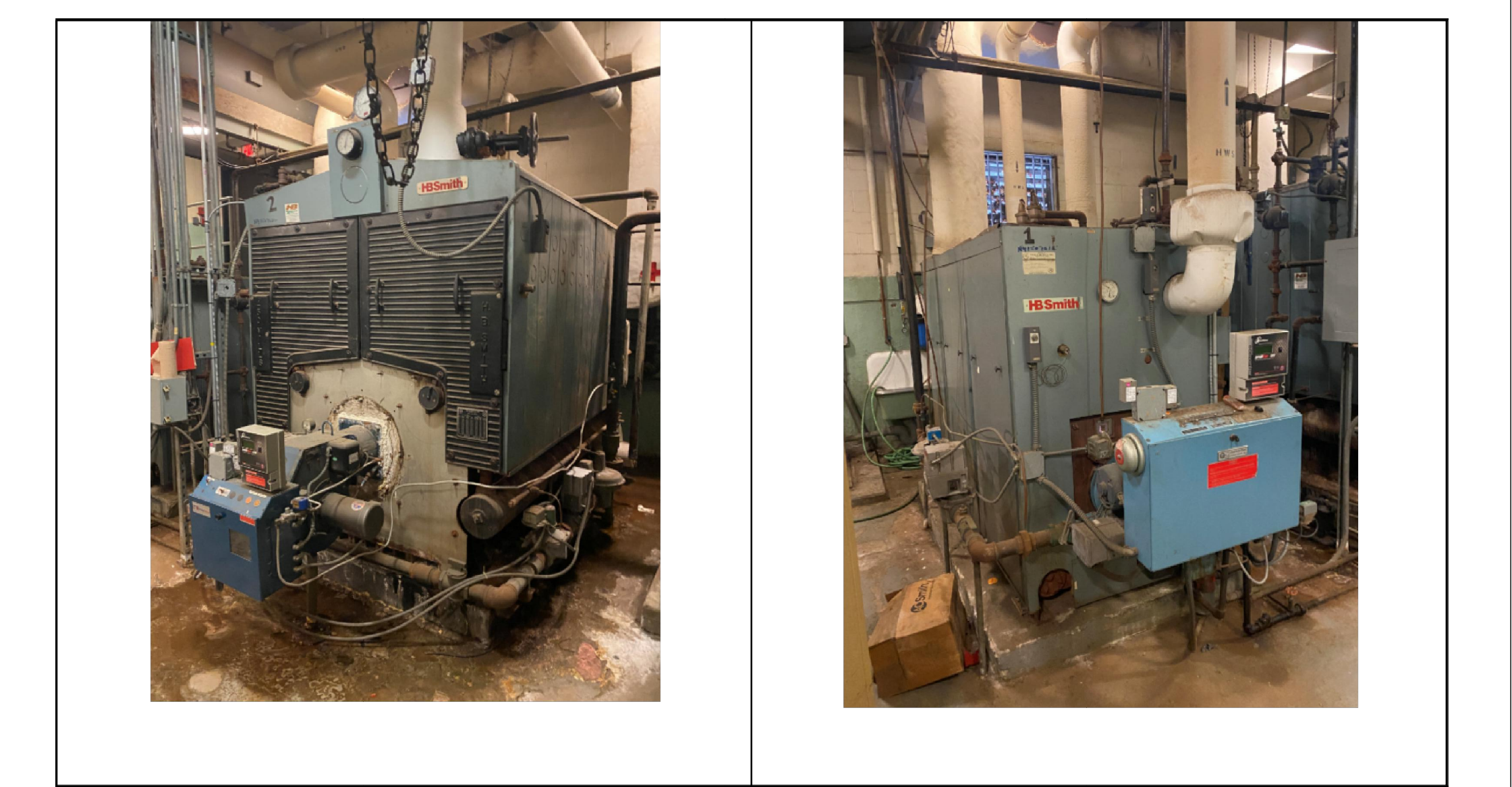
SMITH BOILER TO BE REMOVED
