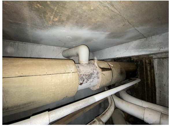
Fiberglass Pipe Insulation with Tar
