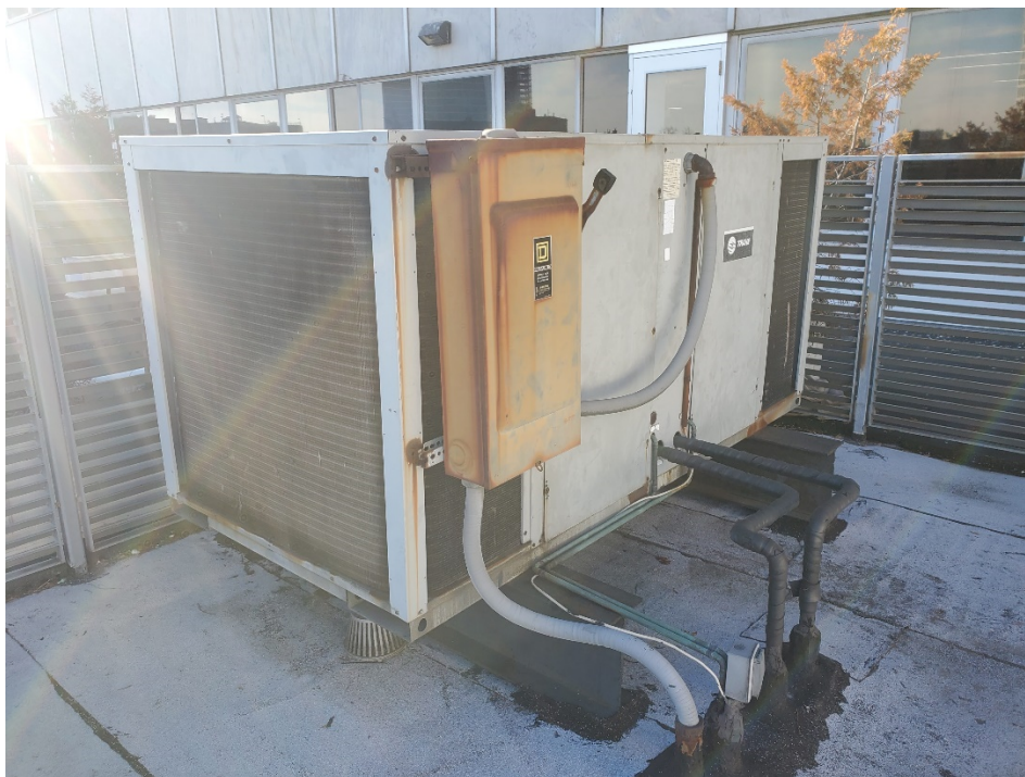
Photo #4 – Condensing Unit on Roof
