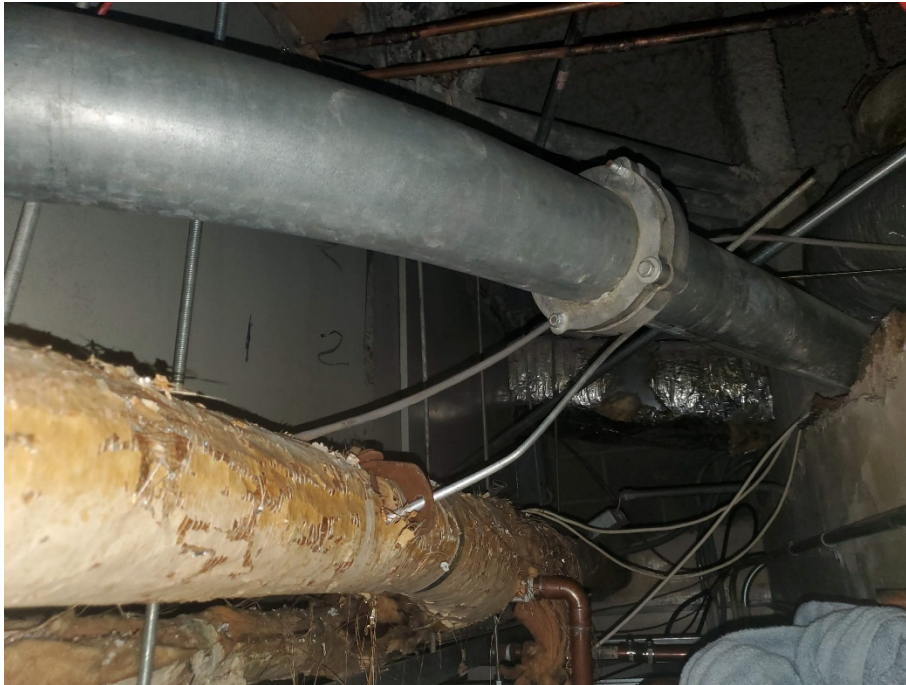
Photo #1 – Existing AHU in Basement Ceiling
