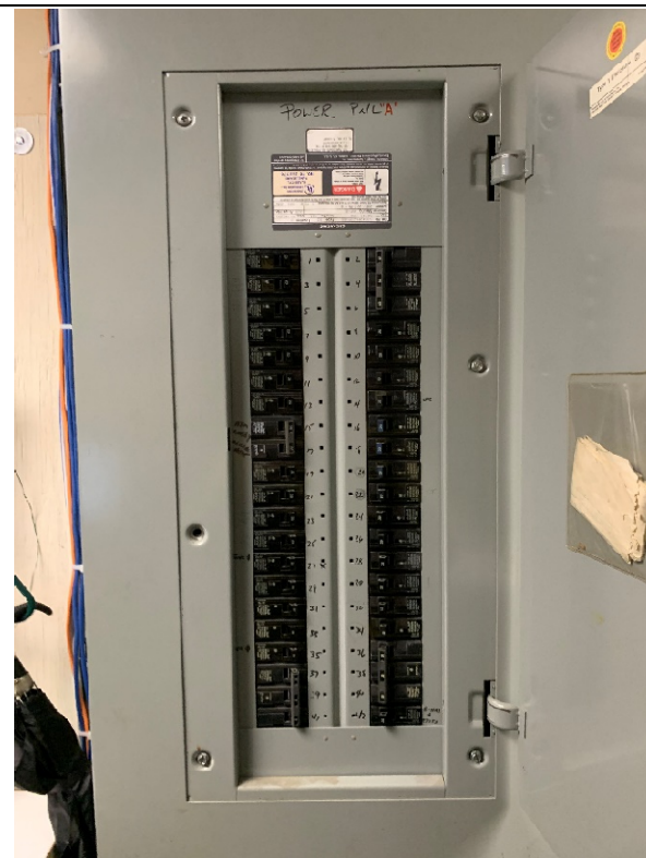
Photo #6 – Panel A Located within Chase Bank Space
