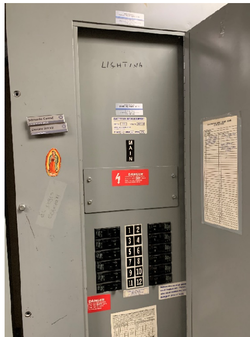
Photo #7 – Lighting Panel Located within Chase Bank Space
