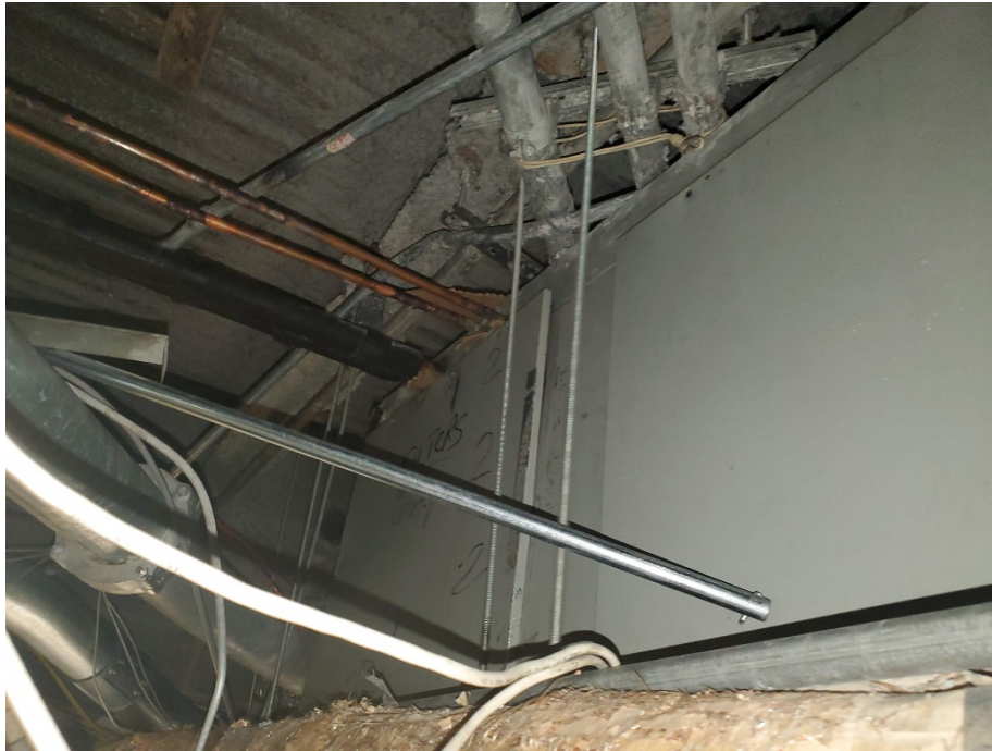
Photo #3 – Blocked Filter Access
