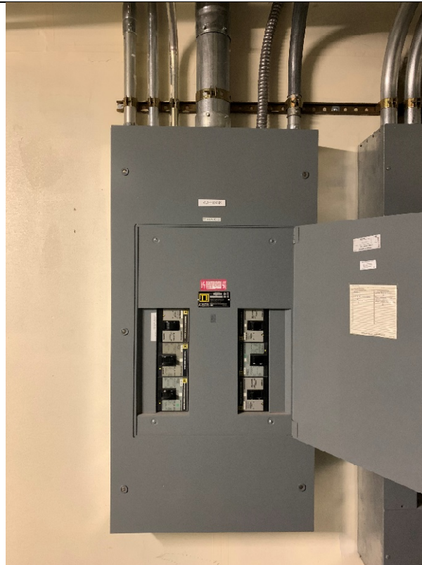
Photo #5 – Chase MDP Located in Base Building Basement Electrical Room
