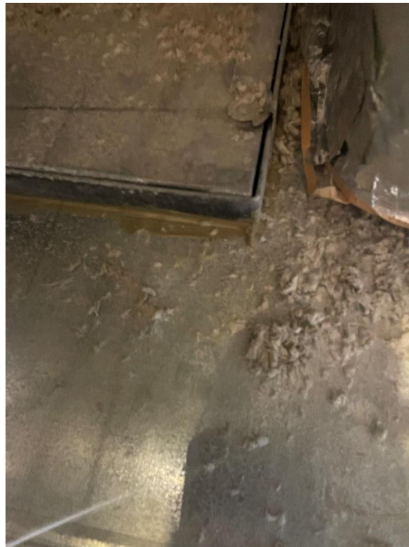
Gold Duct Insulation
