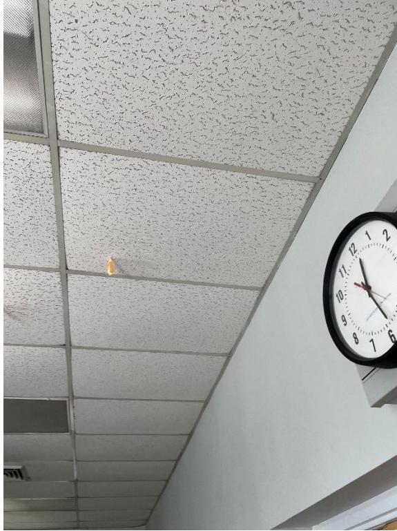
2x4 Fissured Ceiling Tile
