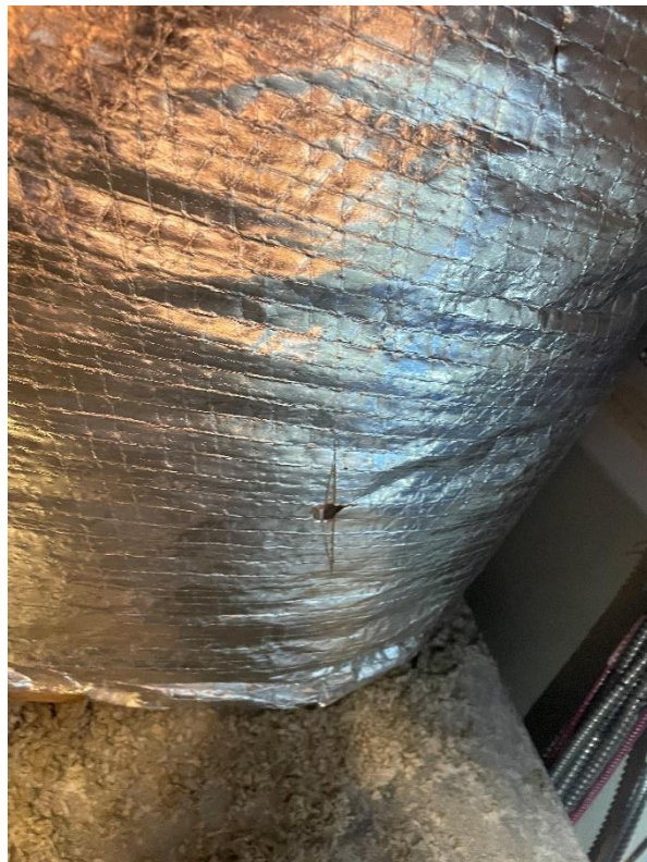
Duct Fiberglass Wrap
