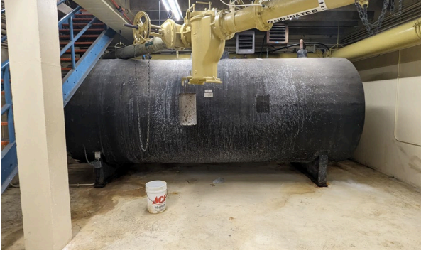
Photograph 1 – 013-01 Black Tank Wrap & 014-01 White Tank Insulation
