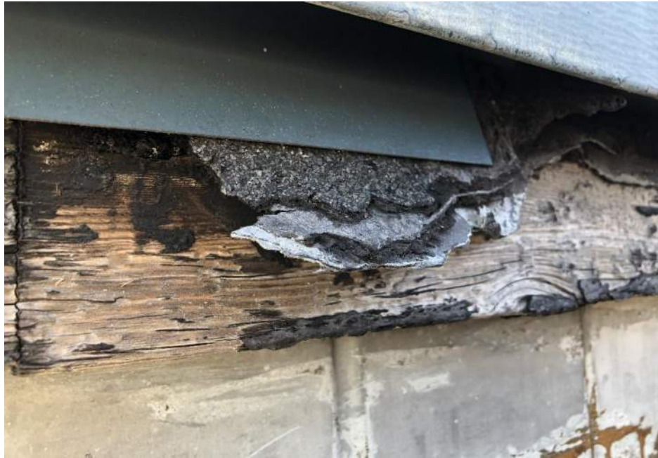
Photo 3 – View of asbestos-containing roofing under the metal cap at the perimeter of the roof on the Transfer Station roof.
