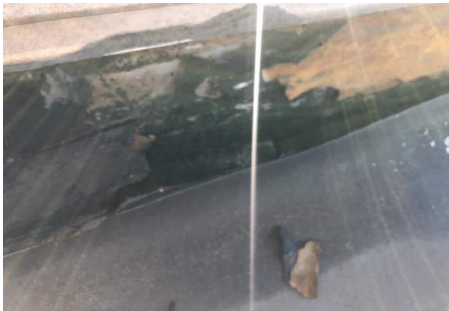
Photo 2 – View of asbestos-containing roof flashing around the skylights on the Transfer Station roof.
